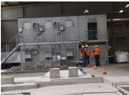
On these foundations, the new rolling mill will be installed. In the back, the afterburner can be seen.
